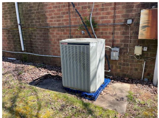
View of HVAC unit
