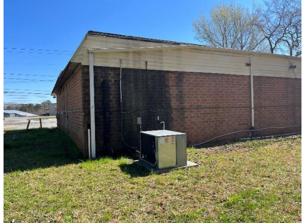
Rear view of the property and potential deferred maintenance
