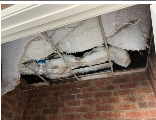
Interior view, ceiling and evidence of roof leaks
