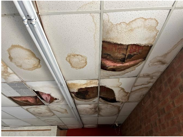
Interior view, ceiling and evidence of roof leaks
